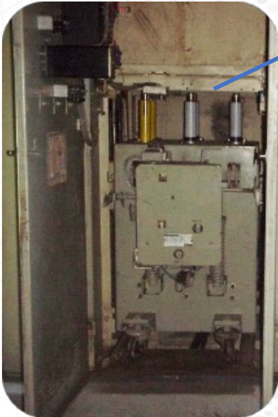
GE MAGNE-BLAST, 1250A @ 13.8KV
